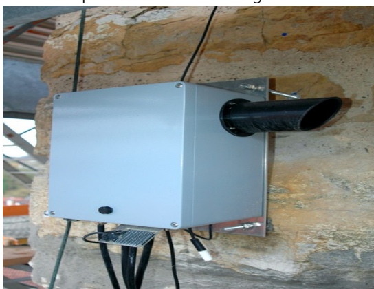
Fig 1: Dimetix Laser Sensor installed at the historical building “Blauer Turm” in Germany
